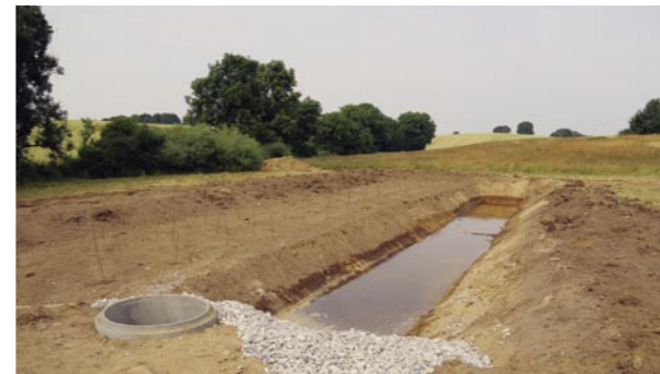
When the buffer zone is set up, a trench running parallel to the stream is created.
